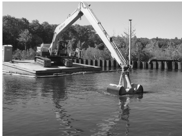
Figure 5. Excavator configured with an environmental clamshell dredge bucket. Note vertical GPS receiver antenna attached to bucket.
